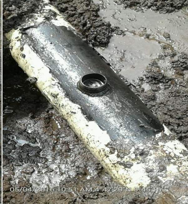
3" Nipple mounted on the pipeline by vandals
